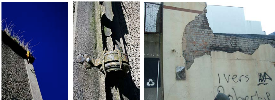
11 (left) Part of a child's scooter suspended on the convent wew wall, Railway Street; 12 (middle) a decaying down-pipe, Gloucester Street convent; 13 (right) exposed brickwork, probably early 20th-century, Foley Street
